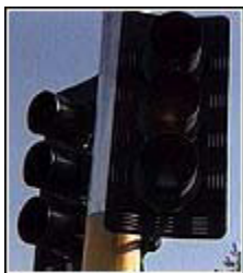
Traffic lights were out in several states (Courtesy KLAS)
